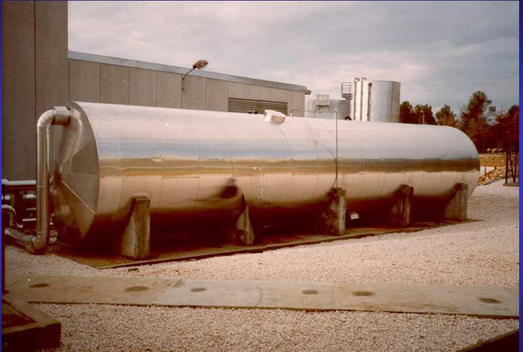
Piping and Tanks Fully Insulated with Jacket
