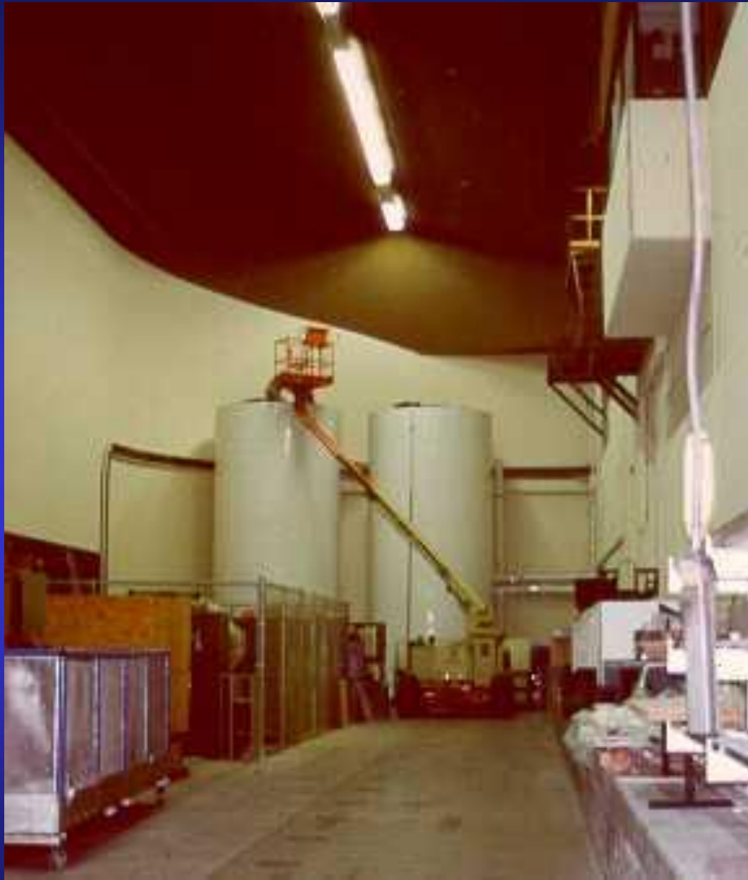
Vertical Atmospheric Tanks Installed Indoors
