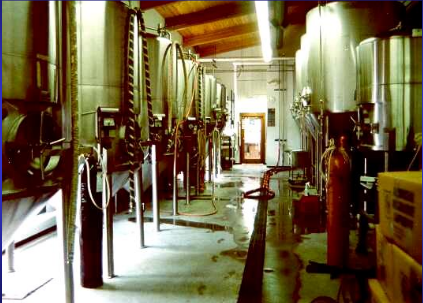
Brewery Tanks with Cooling Jackets
