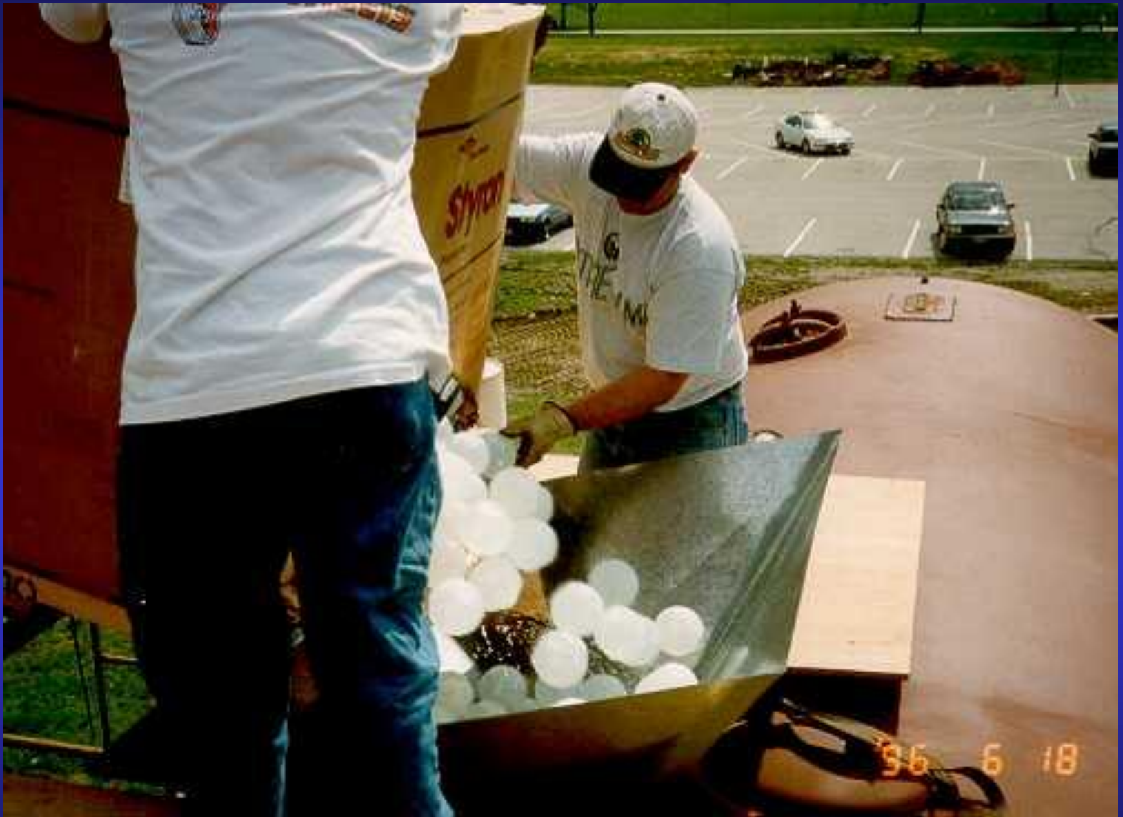
Pouring Balls Into Tank - Tank is 2/3 Full of Water to Aid Installation
