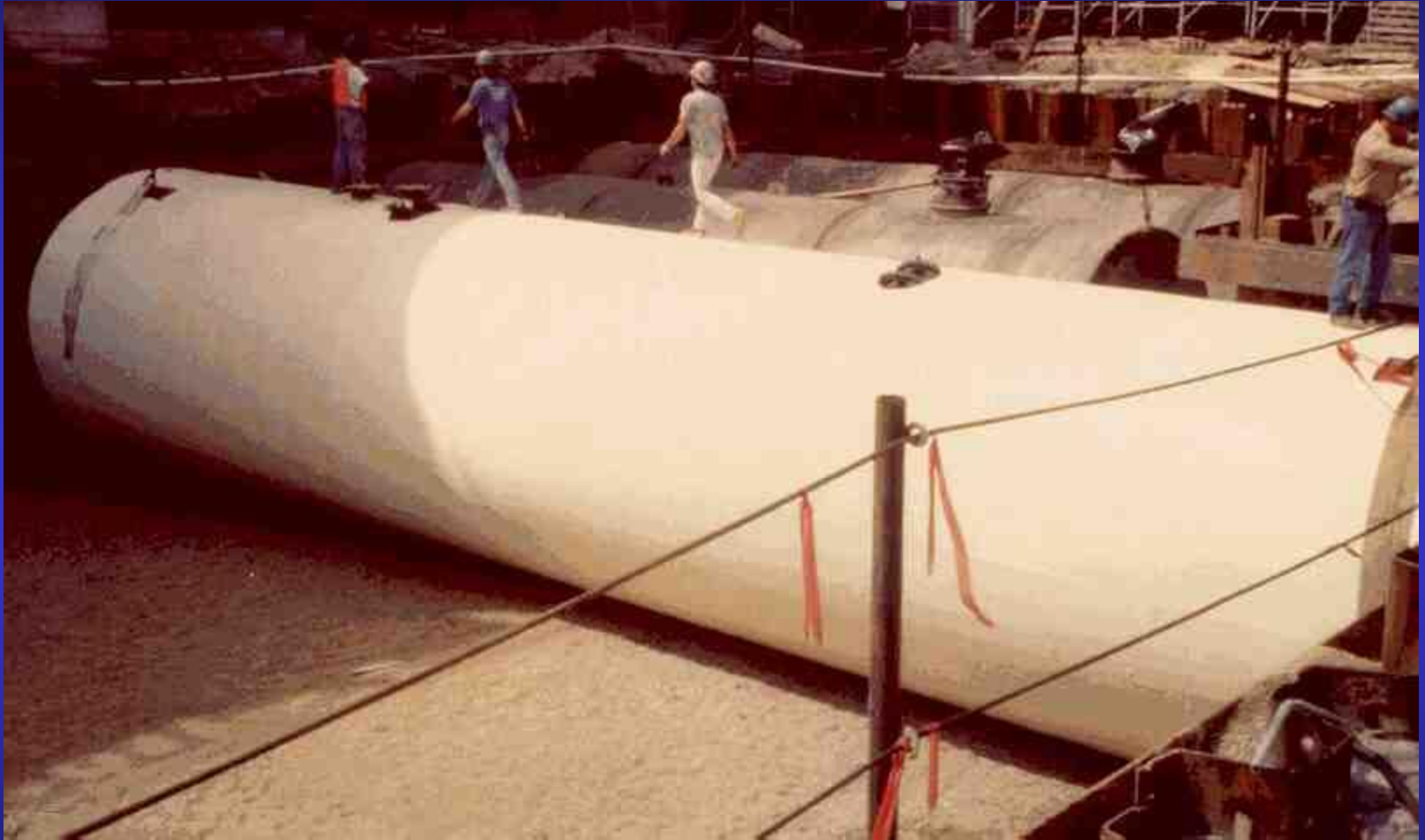
Horizontal Pressure Vessel - 2,500 Ton Hours per Tank
